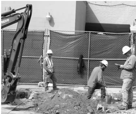
Below: Electrical work with excavation and new vaults taking place in the parking lot east of Harbor. Flowerbeds are also being upgraded.
